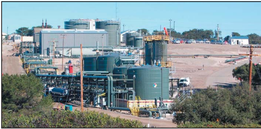
Photo 4. New facilities, tanks, and a reverse osmosis system were installed in the Orcutt oil field to handle the increased activity and production. Photo by R. Brunetti.
