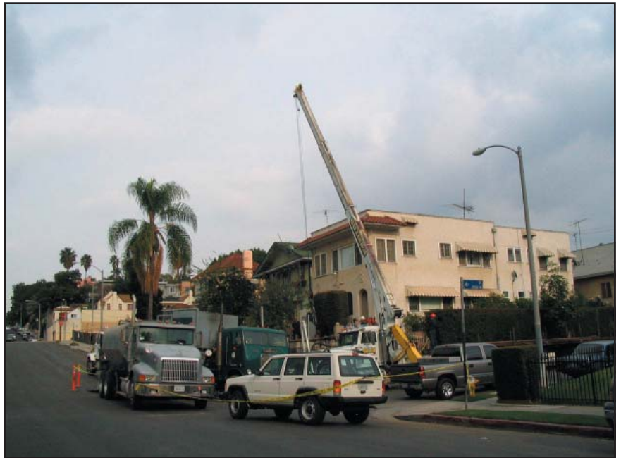
Photo 5. Well L.A.R.R. Co. 1A. The street is temporary blocked with equipment while the well is plugged with cement. Photo by C. McCullough.
