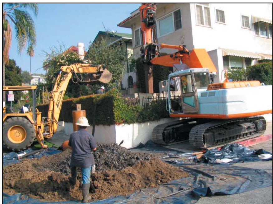
Photo 4. Well L.A.R.R. Co. 1A. Auger and backhoe were used to clean out the well. Photo by G. Brandt.
