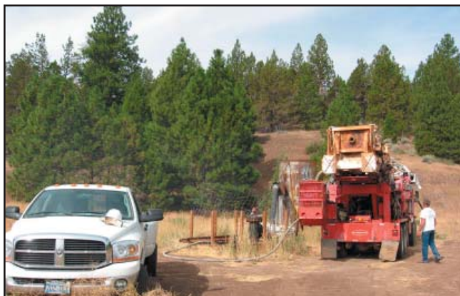
Mechanical integrity test of idle geothermal well "Phipps" 2 near Cedarville. Photo by J. Truschel.
