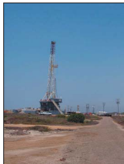
Kenia Rig # 6 drilling well "State PRC 3314" F-2 in the West Montalvo Offshore field. Photo by district staff.
