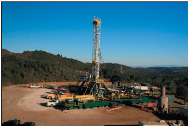
ThermaSource rig 105 drilling at Bottle Rock Power LLC's well "Coleman 7-6." This is the first rig at The Geysers with automatic hydraulic pipe-handling. In the background is rig Kenai 6 drilling well "California State 92-6" for Geysers Power Company, LLC. Photo by W. Leuzinger.
