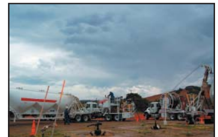
Photo 6. Using a conventional workover rig, contractor Nabors Well Services plugged and abandoned wells for Chevron USA Inc. in the Cat Canyon oil field. Photo by R. Brunetti.
