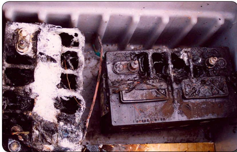
Batteries, like these conversional wet-cells, have always had the potential to start fires due to their high energy content. These caught fire when an errant wrench contacted both terminals (Claim #0205712). Newer technology batteries with higher capacities and less forgiving charging characteristics will require even more caution along with sophisticated monitoring.
