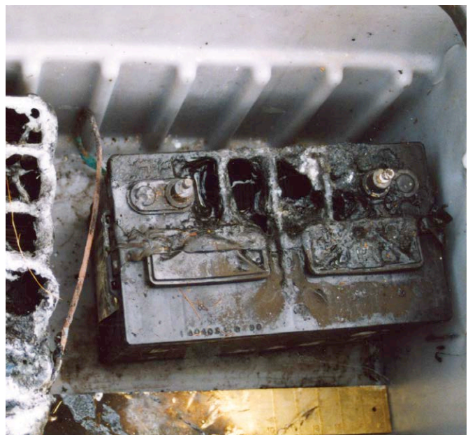
Reconnecting battery cables incorrectly can cause all kinds of havoc in the electrical system, including a fire.
