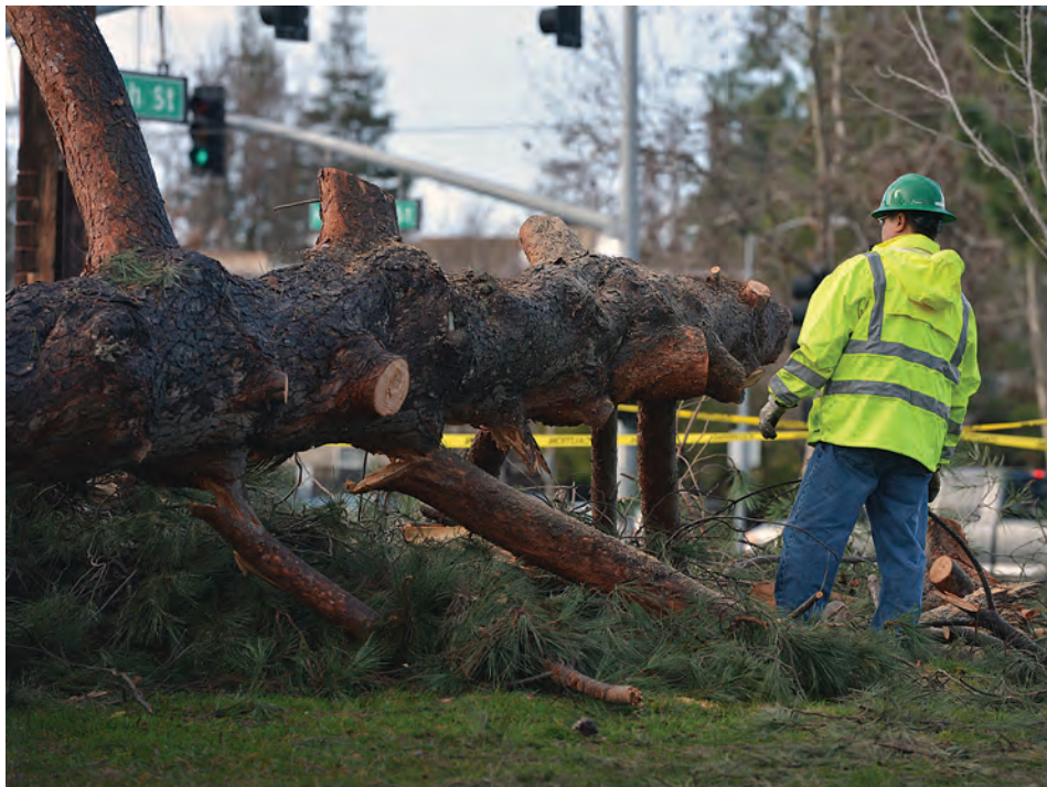
Work crews worked to remove a large tree that was uprooted during the recent storms. The tree was located at Centennial Park on the northeast corner of 4th and Holmes.
