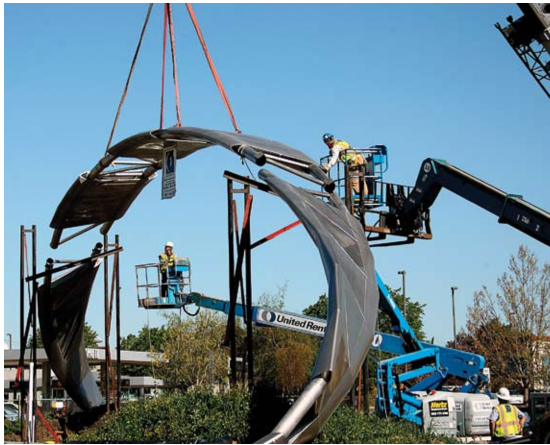
Workers from Ogletree Inc. installed the centerpiece of the City of Dublin's new gateway feature, "The Eternal Ribbon." Funded completely with federal transportation dollars, the Eternal Ribbon is a twisting stainless steel arch that spans 100 feet long and 22 feet high. The sculptural arch is intended to give people the experience of passage, and when viewed from above, is the symbol for infinity. The project is part of a larger Corridor Enhancement project that will also include the installation of new gateway markers and monument and directional signs along Dublin Boulevard.
