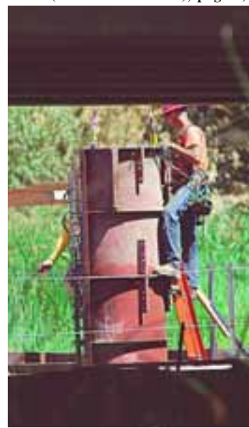
Work is underway on a bridge over the Arroyo Del Valle in Pleasanton. The project includes the construction of a second bridge on Bernal Avenue near Vineyard Avenue. It will allow for two lanes in each direction and the widening of Bernal Avenue to the bridge. Funds will also go toward installing a sewer line and the creation of wetland and riparian habitat in the arroyo to mitigate construction impacts.
