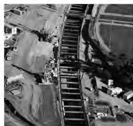
Funded in part by Measure B, the BART Warm Springs Extension is the beginning of a new connection to Silicon Valley and has employed hundreds of local workers.
