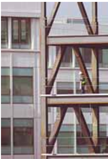
Workmen were busy constructing new facilities at Oracle in Pleasanton, at the same time creating patterns of light and shadow.
