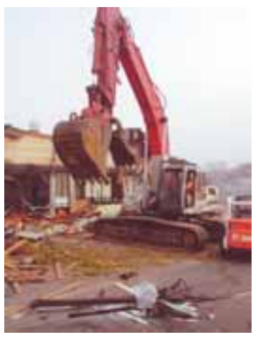
Photo - Doug Jorgensen Crews began knocking down the old Lucky Store on Railroad Avenue in Livermore last week. The city is looking at new uses for the land, including a 2000-seat regional performing arts theater and housing along with some retail. The two businesses still at the site will remain there until they can be relocated. City officials recently interviewed five companies seeking to build a mixed use project in conjunction with the theater.
