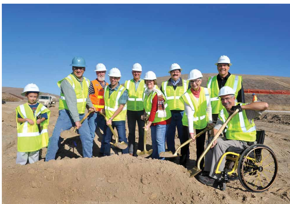
A ground-breaking ceremony was held last Friday to signal the start of the construction of Cayetano Creek Park in North Livermore. Pictured are (adults, from left) LARPD Vice President David Hutchinson, Project Manager Larry Kerbs, Land Development Purchasing Agent Brady Stephenson, Shea Properties Vice President Jeff Melrose, LARPD President Maryalice Faltings, LARPD General Manager Tim Barry, LARPD Director Beth Wilson, LARPD Assistant General Manager John Lawrence and LARPD Director Bob Coomber. The park has an anticipated opening date in late fall 2014. It will include a synthetic turf field, tot lot, dog park, restrooms, basketball court, a grass practice field and picnic areas. Photo - Gina Halferty for LARPD
