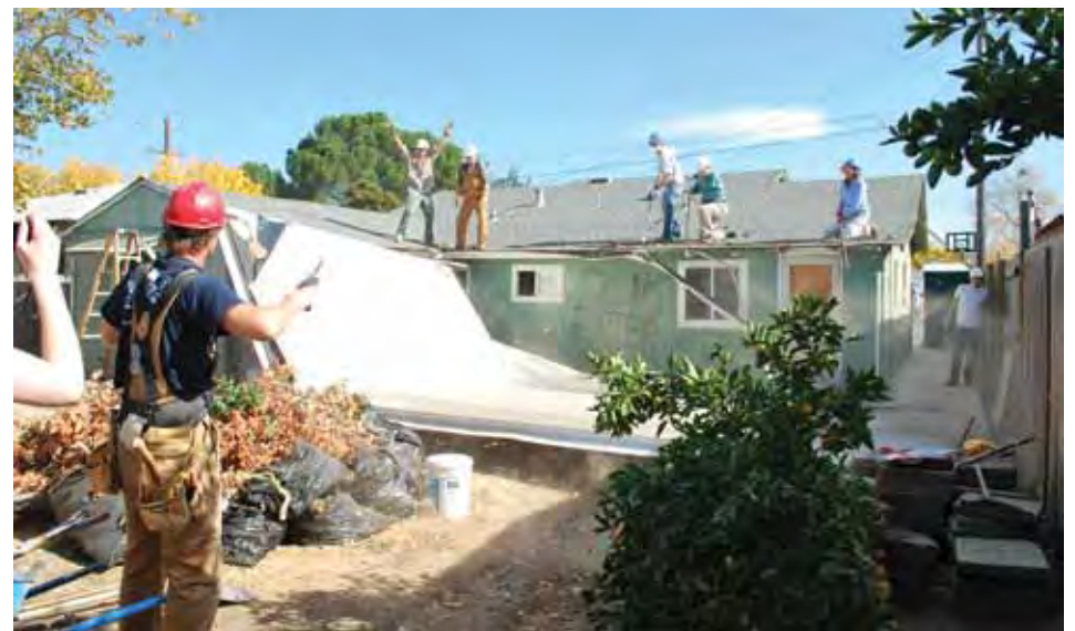
A crew of Sandia volunteers cheers after safely collapsing the outdoor patio roof of a Habitat home that they would soon rebuild. (Photo by Catherine Dawson)
