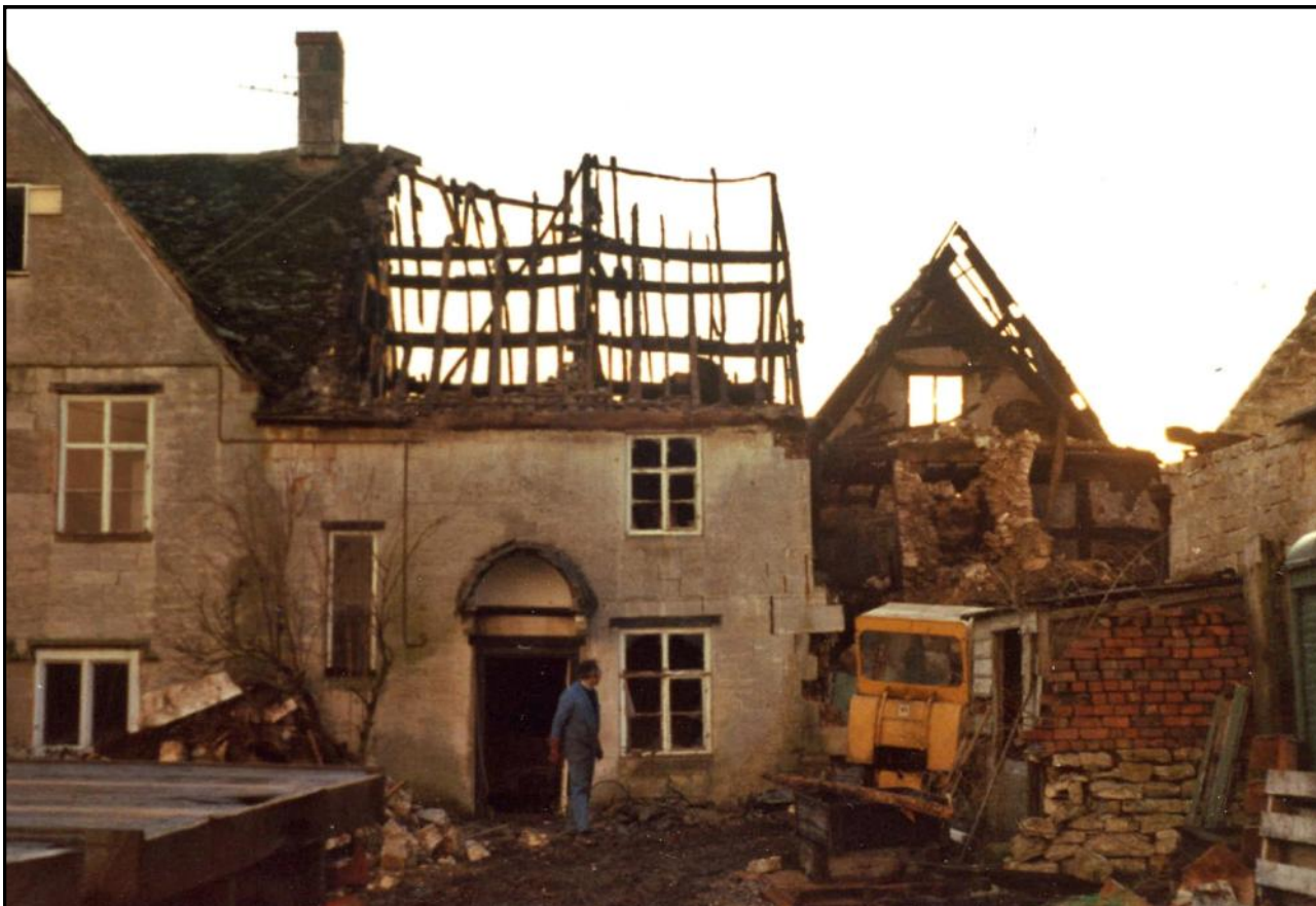
Oldends Hall from the north-east after the fire, showing the damaged roof timbers of the medieval hall and extended service block.
