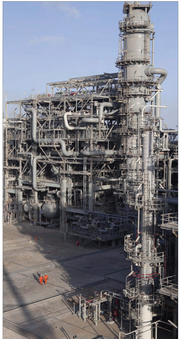
Qatargas 2 Trains 4 and 5 both began operations in 2009 and have a combined design capacity of 15.6 million tonnes of LNG per year.
