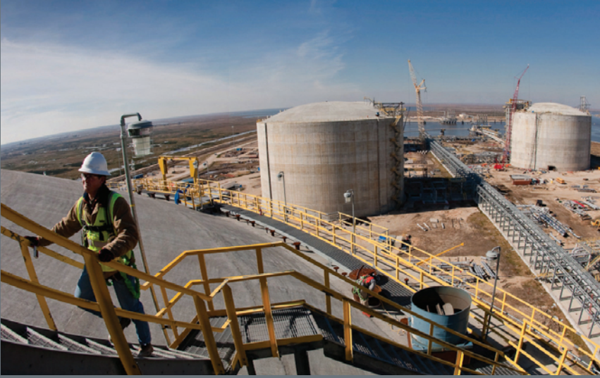
The Golden Pass LNG regasification terminal, located on the U.S. Gulf Coast, will open in 2010 and will have the capacity to supply 2 billion cubic feet of gas per day to the U.S. market.
