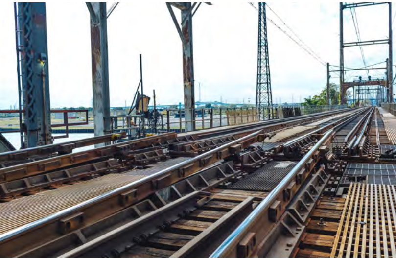
The Portal Bridge's "Miter Rails" (center) are the source of many delays.
