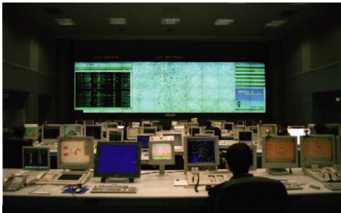
Communication Command Center
