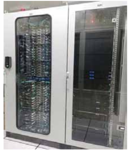
Computer/ Server Racks of HPC
