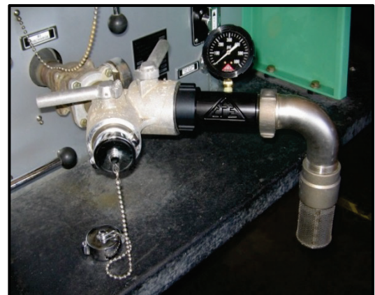
Figure 10. Pressure valve attached to the footvalve.
