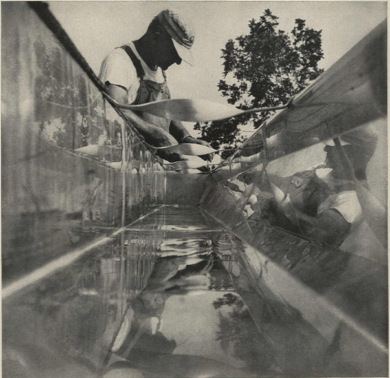
Installation: Sts. Philip and James School-Church-Auditorium, St. James, New York. Architect: John O'Malley and Associates. General Contractor: Schumacher & Forelle, Inc. Roofing: John Schneider Roofing Contractors, Inc.
