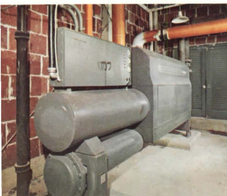
J. This 137-ton PE direct expansion packaged chiller fits through a 30-inch door. Installed in three-story addition to the Sheffield Memorial building, Atlanta, Ga., it is completely factory assembled, pretested and charged. Also included in job are Westinghouse-Sturtevant fans and air handling equipment.
