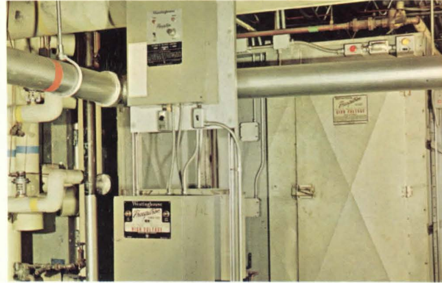
D. Westinghouse Precipitron® electronic air cleaner removes up to 95% of all dirt particles, smoke and pollen circulating throughout a building. Traps particles as small as 1/100th micron. Holds contaminants on electrically charged plates, without reducing flow of air through the cleaner.
