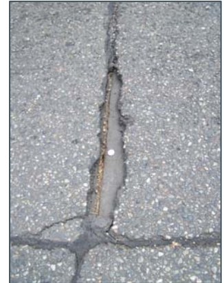
Bicycle spot improvements can fix pavement problems.
