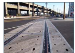
Inactive railroad tracks on Alaskan Way S where flange fillers have been used.
