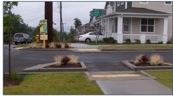
Curb extensions were constructed on SW Juneau Street to slow motor vehicles.
