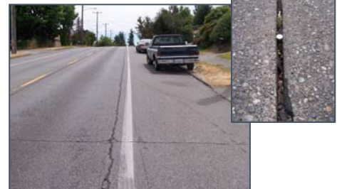
This seam on Renton Avenue S is approximately one inch wide in some places.
