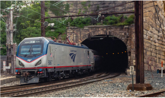
Amtrak completed concrete slab, tie and rail replacement work at the Baltimore & Potomac Tunnel, which opened to train traffic in 1873 and is located west of Baltimore Penn Station.
