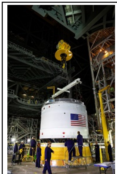
Shown here are engineers integrating NASA's Space Launch System (SLS) rocket with the launch vehicle stage adapter (LVSA) at Kennedy Space Center's Vehicle Assemble Building (VAB) using advanced cranes and unique mechanical systems.
