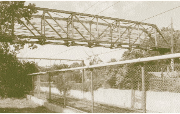
left: A number of footbridges were constructed over the cut, or approach to Boston, to connect the bisected areas. In Forest Hills, the tracks are crossed by the Mount Hope Footbridge, a 75-foot long, steel-truss structure built about 1910. PAL
