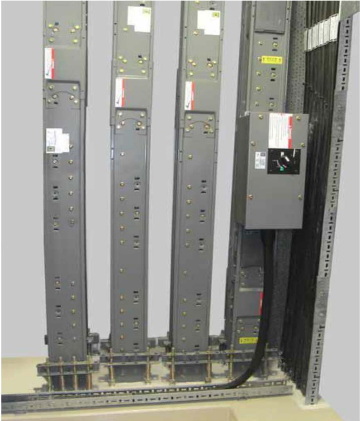
Typical busbar riser system including plug-in circuit breaker
