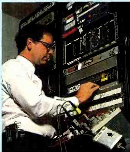
On October 15, 1984 at KTLA’s Mt. Wilson transmitter site, Ira Goldstone performed the final acceptance checks on the Modulation Sciences TV. Stereo Generator.
