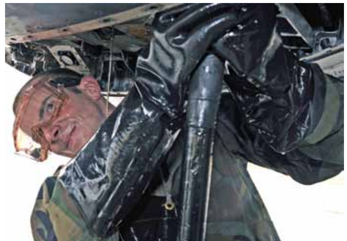
A1C Derrick Gregg removes a hydraulic test line from a B1-B Bomber.
