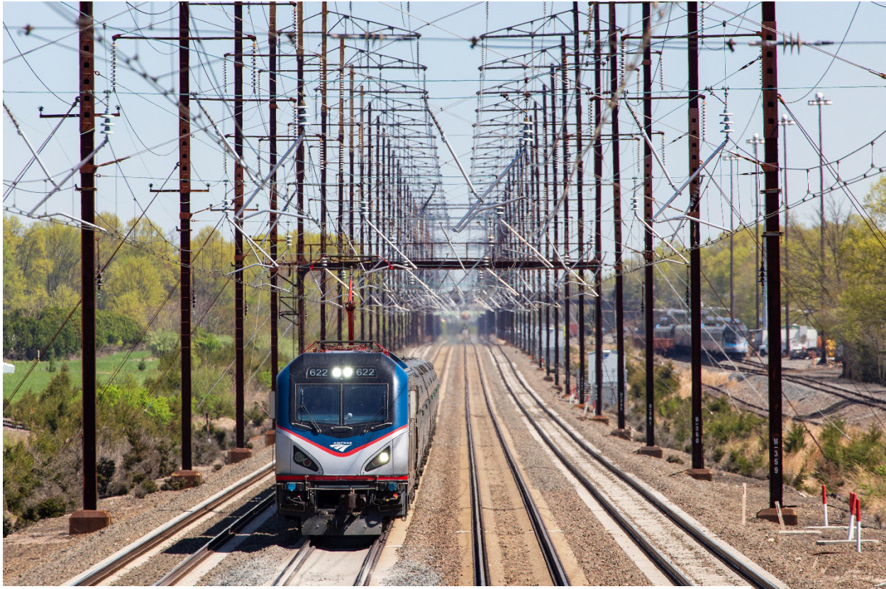
Catenary Lines in New Jersey
