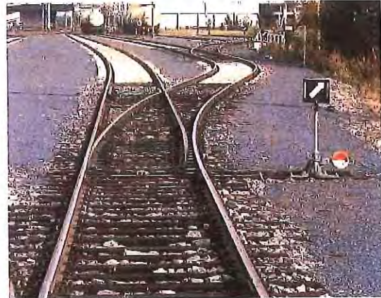
Figure 15. Turnout Track Example (Teve, 2006)
