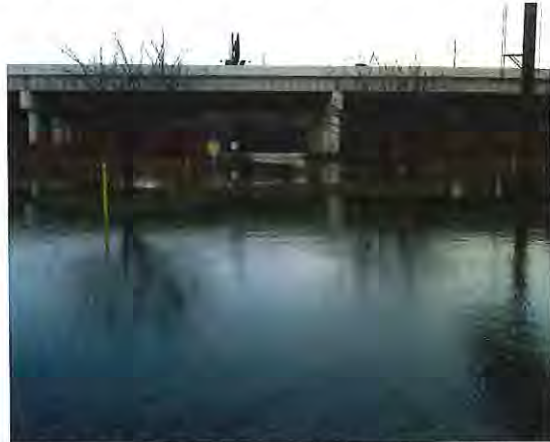
Figure 44. Example of Flooding to the Parking Area at the Wilmington Training Center Flooding
