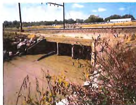
Figure 12. Perkin Creek Bridge located within the Pilot Study Area (b) (5) Example of bridge crossing water (photo source: Amtrak)
