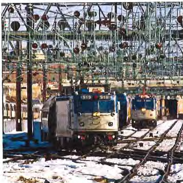
Figure 43. "Constant-tension" Catenary System ( NEC Commission, 2015)
