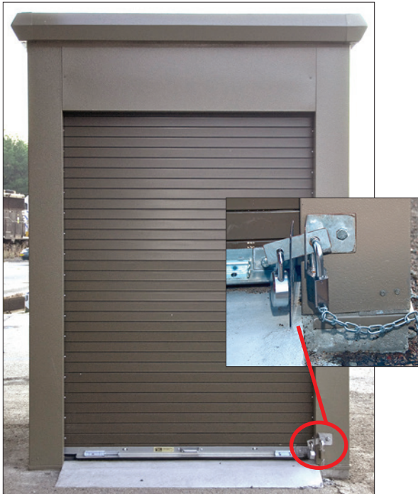
Figure 11-8 – Example of Shed with Locks in the Correct Position
