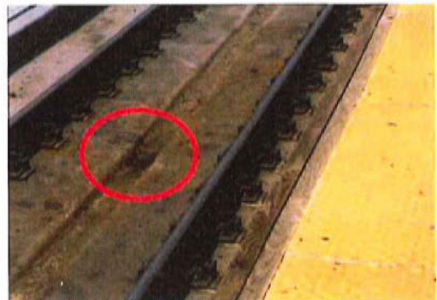
Figure 7. Water Infiltration between the Rails
