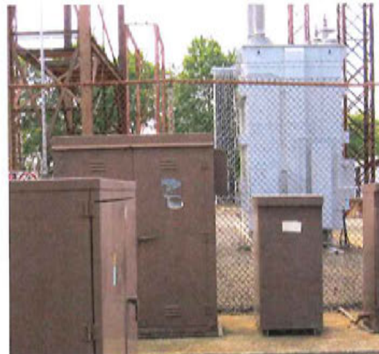
Figure 36. West Yard - Substation Equipment
