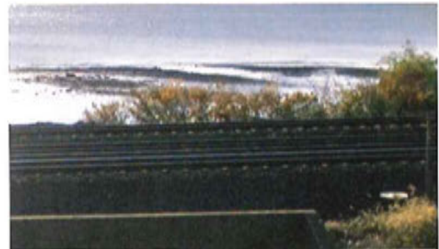
Figure 44. Rail Ties and Ballast above Culvert Discharging into Delaware River (MP 21.0 to 21.5)
