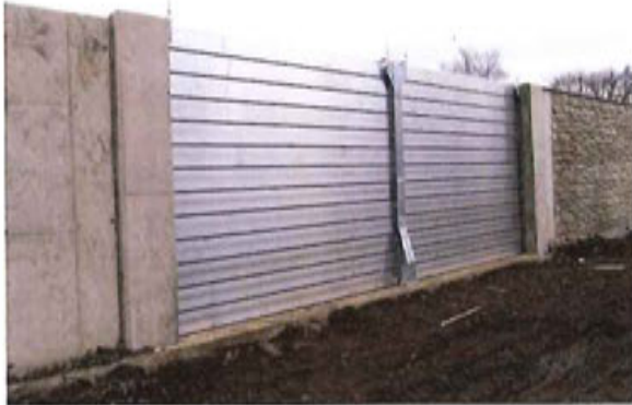
Figure 39. Permanent Concrete Flood Wall
