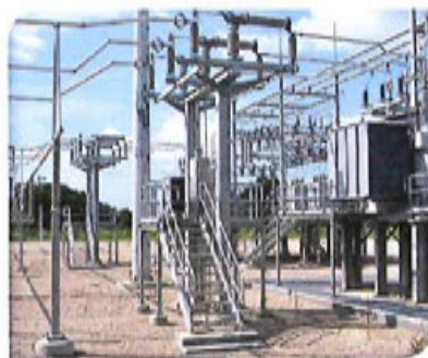
Photo Credit: DIS-TRAN Packaged Substations (distransubstations.com)
