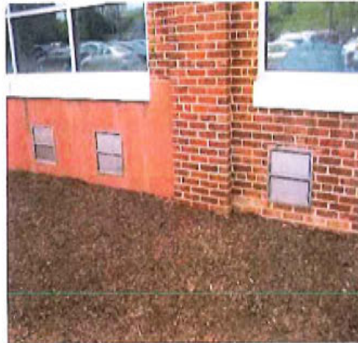
Figure 24. Flood vents located below the first floor.
