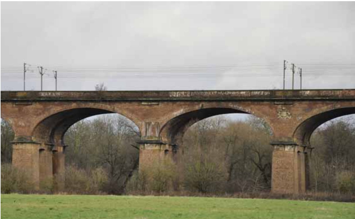
Wharncliffe Viaduct, Great Western Main Line (Grade I). OLE installed c.1998 (photograph: ©Alan Baxter & Associates)
