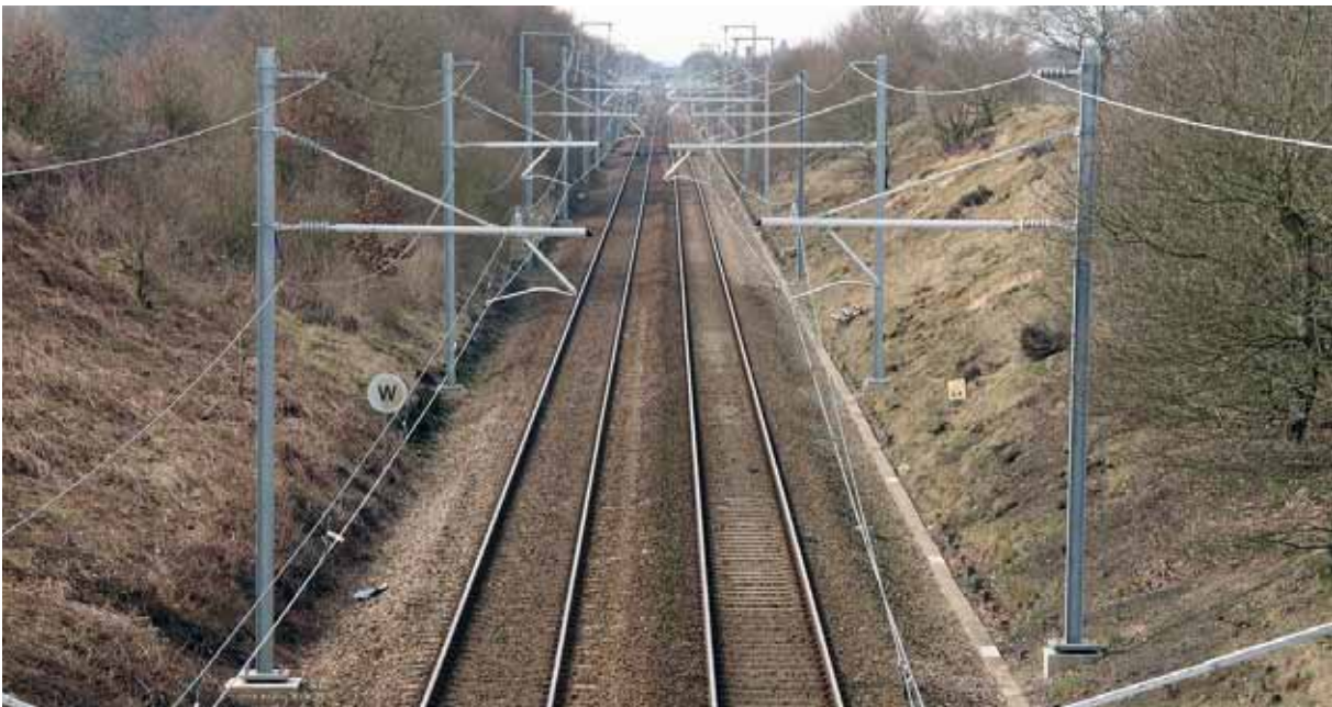
Newly installed Series Two OLE cantilever masts on the North West Electrification Project (photograph: ©Mark Barber)
