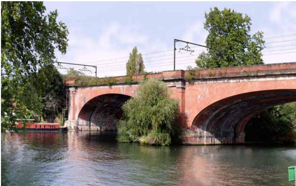
Maidenhead Railway Bridge, Great Western Main Line (Grade I). Proposed OLE supports (photograph: ©Network Rail)
