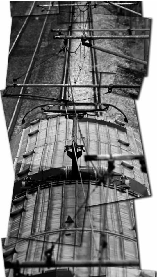
Stagger of contact wire and catenary. Note also the pantograph on top of the train (photograph ©Graeme Bickerdike/Four by Three)
