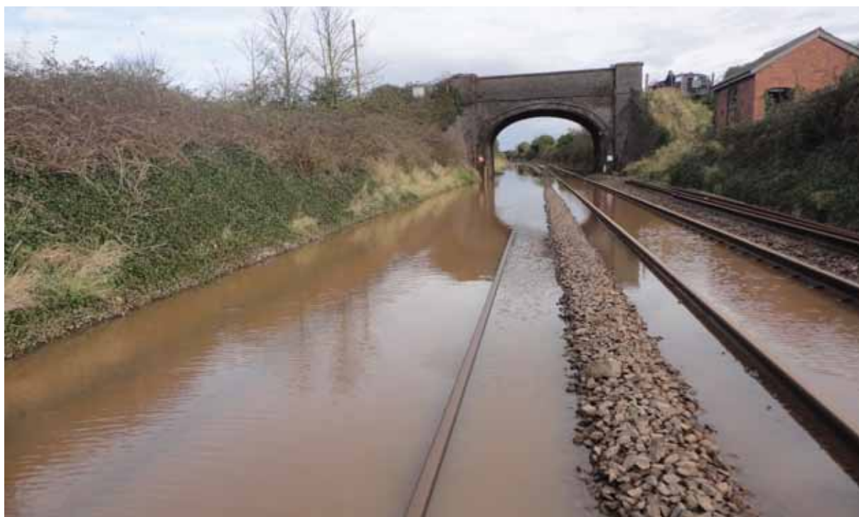
Water collecting at low points on the track causes many thousands of 'delay minutes' each year (photograph: ©Network Rail)
