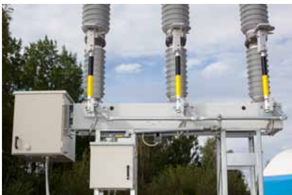
Earthing switch in closed/earthed position.
