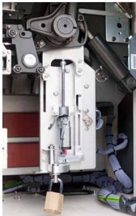
Disconnecting circuit breaker in blocked and padlocked position.
