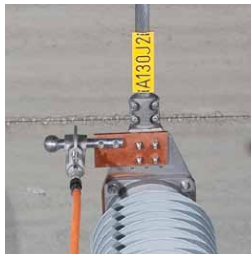
Earthing device connected to phase terminal
