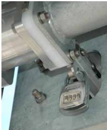
Blocking activated and padlock applied.
