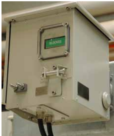
The disconnecting circuit breaker is blocked in open position. The sign indicates blocked.
