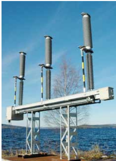
Earthing switch in earthed position.
