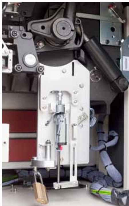
Disconnecting circuit breaker unblocked in open position.
