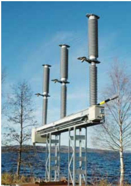
Earthing switch in unearthed position.
