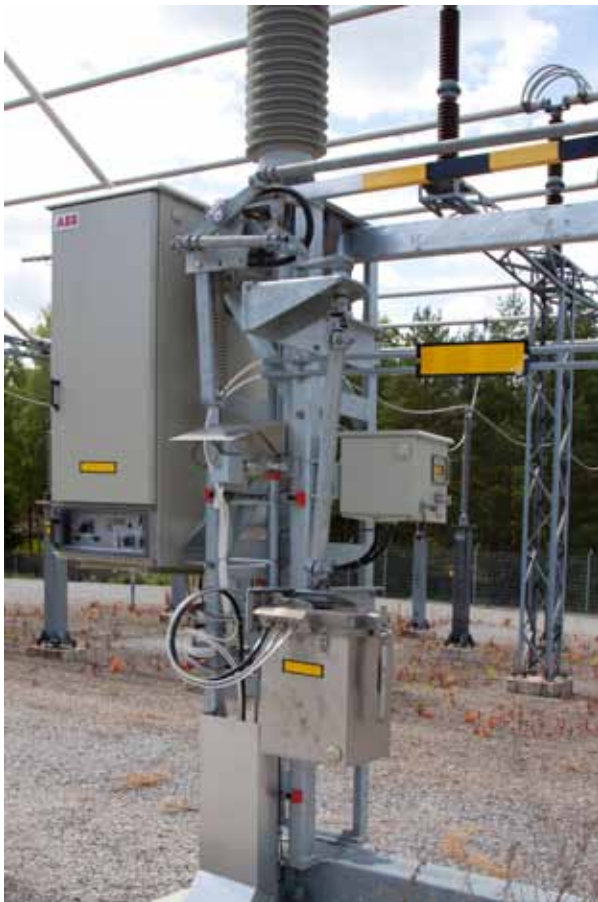
Earthing switch in open position.
