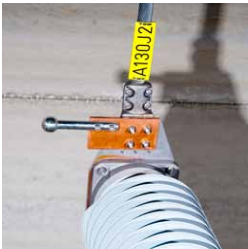
Phase connection terminal
