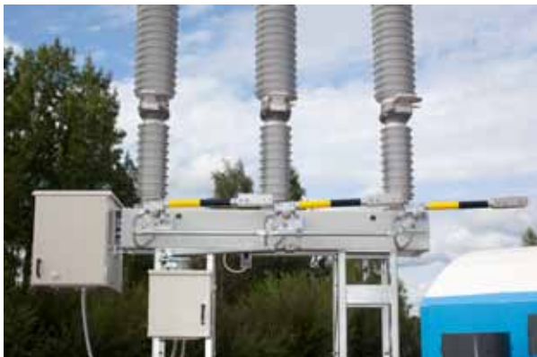
Earthing switch in open position.
