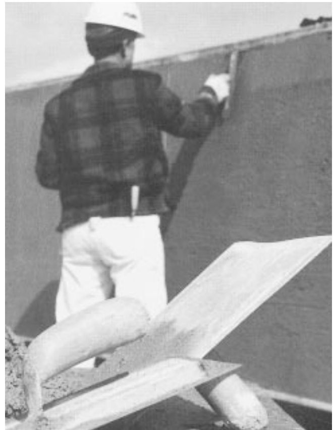
Figure 1. A plasterer trowels a wall face. Flat wall surfaces are some of the simplest and most common plaster applications. (30241-0)
