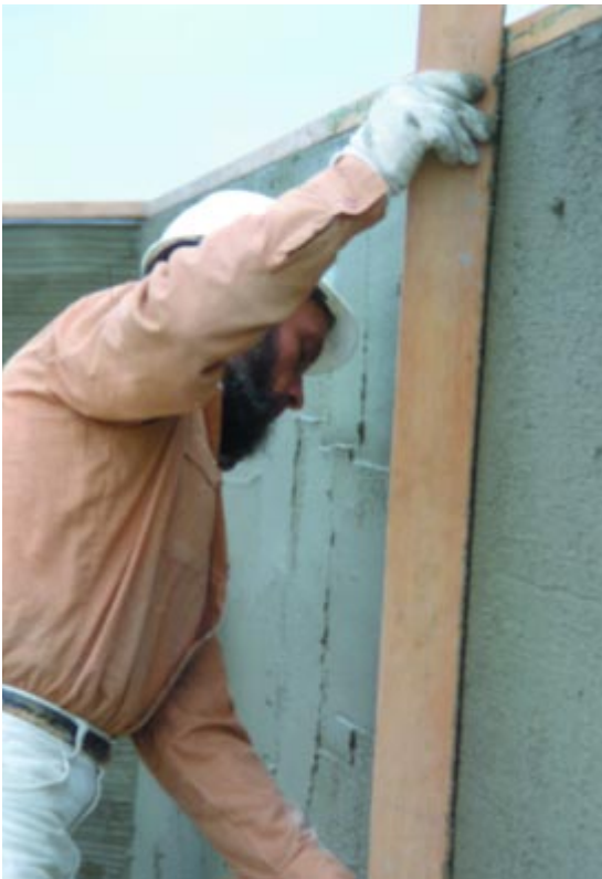
Figure 20. A few minutes after the brown coat is applied, the surface is rodded to the desired plane. (70208)
