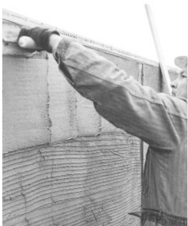
Figure 19. The second (brown) coat is applied in a thickness to bring the surface to the proper plane. (30241-D)
