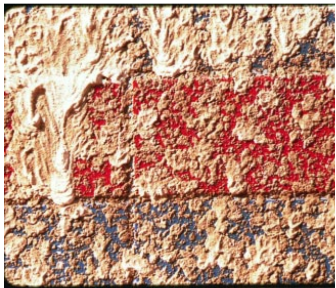
Figure 5. A dash-bond coat can be applied to enhance bond between a solid base and plaster. (40630)
