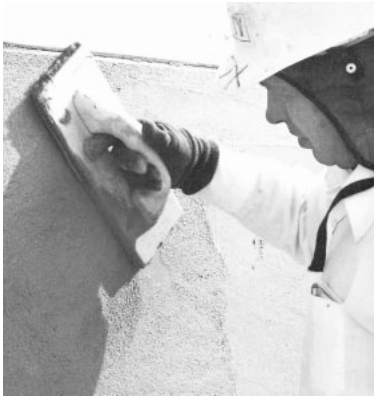
Figure 21. Finally, the finish coat is applied to a predamped, but still absorptive, brown coat and floated and textured to the desired finish. (30241-J)
