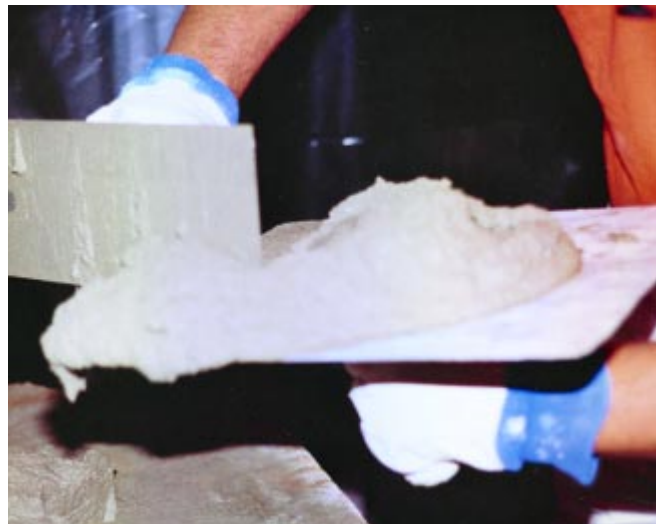
Figure 17. The plasterer takes plaster from the board, puts it on his hawk, and begins to plaster the surface. (IMG12629)
