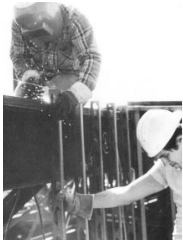
Figure 8. Metal studs should be properly spaced and securely fastened to structural steel. (30570-J)
