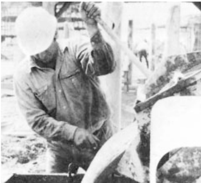
Figure 15. Plaster pump is placed adjacent to the mortar mixer to deliver the plaster to the work area. (30570-K)
