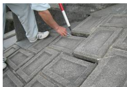
(取付護岸の沈下と空洞)
