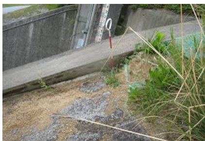
(胸壁と取付護岸のズレ)
