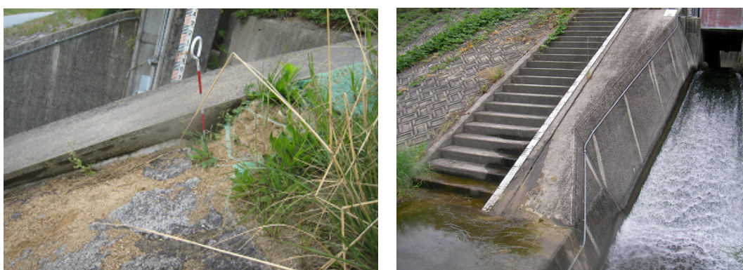
(樋門の胸壁と取付護岸のズレ)
