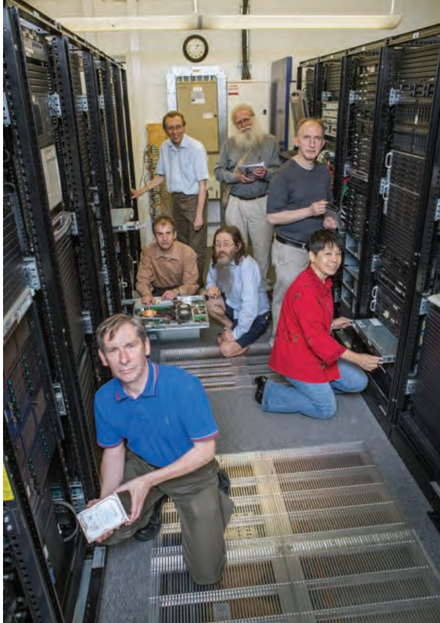
The Computer Officers, seen here in a server room, are responsible for maintaining and extending the infrastructure supporting the research, teaching and administration of the Computer Laboratory. Some are also involved in research and teaching. From the back, left to right in all cases: Graham Titmus, Robin Fairbairns (standing), Martyn Johnson, Pieter Brooks (kneeling), Chris Hadley (standing), Jiang He and Brian Jones (kneeling).
