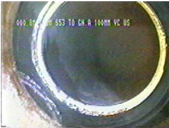
Plate F7 Open Joint Displaced over 1.5x Pipe Wall Thickness
