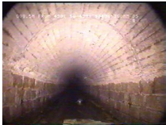
Plate F8 Spalling of Pipe Wall
