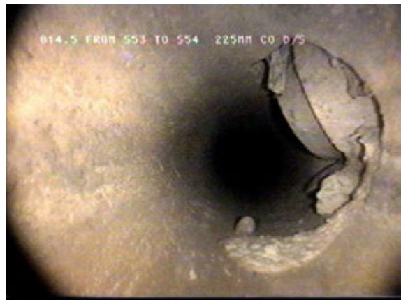
Plate F10 Connection Defect with Intruding Pipe
