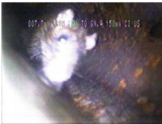
Plate F21 Vermin Encountered in Pipe
