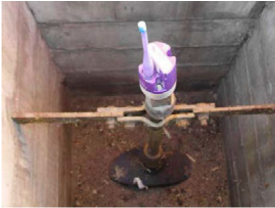
Plate H5 Noise Logger in a Valve Chamber
