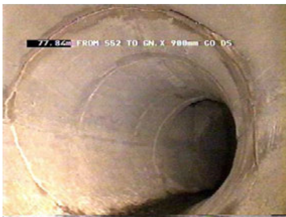
Plate F17 Line Deviation of Pipe to the Right
