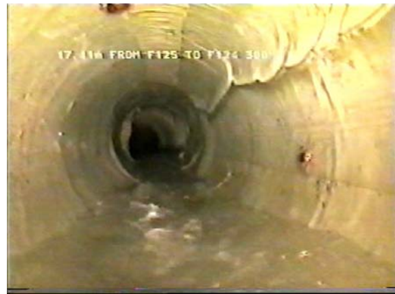
Plate F20 Bulging of Pipe Lining
