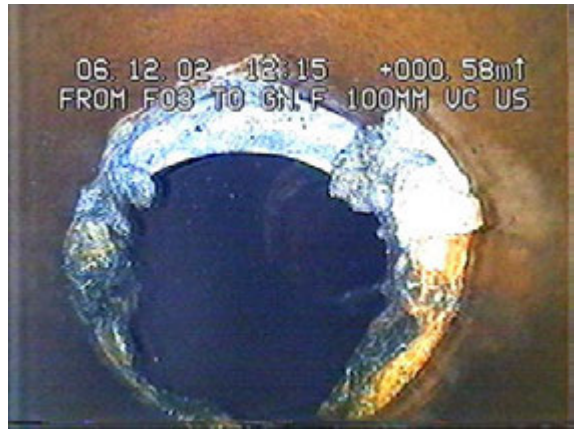
Plate F16 Heavy Encrustation on Pipe Wall
