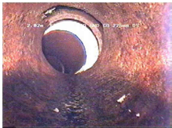
Plate F6 Joint Displaced over 1.5x Pipe Wall Thickness
