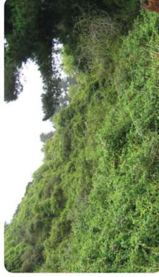
6. At approximately Chainage 3750 (the Area marked as A3 in the above Engineering drawings), the vegetation affected is a mix of low shrubs and contains a large number of weed species such as blackberry. The native species further up the slope will largely be unaffected by the proposed works.
