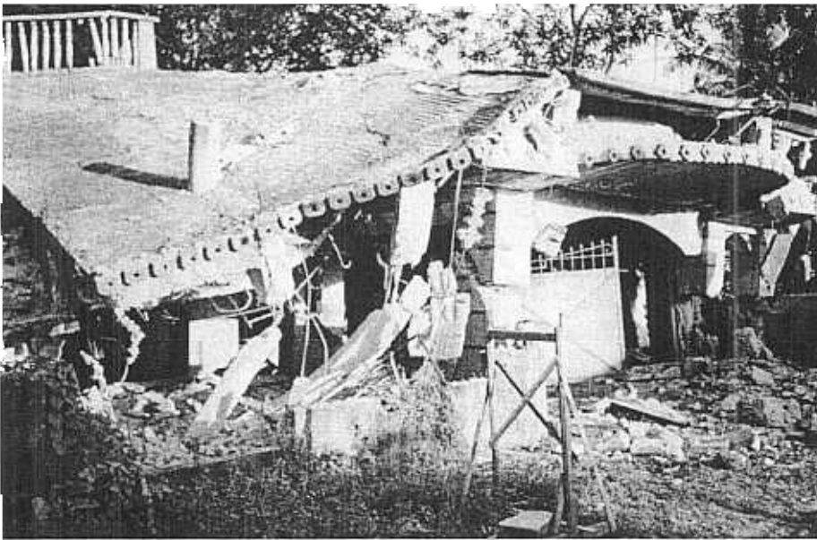
Feb. 8, 1990. Bohol Earthquake. A 2-story reinforced concrete building at Guindulman, Bohol collapsed during the 2nd shock. A column punched through the slab.
