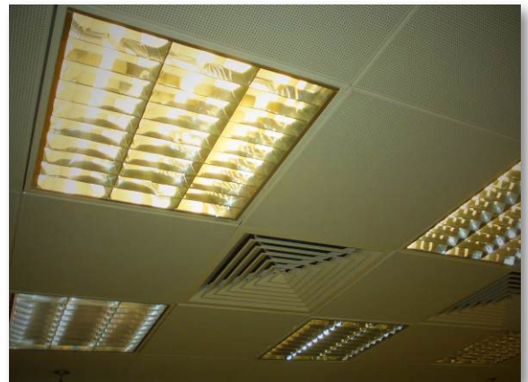
Retrofittings by electronic ballast at HAHQs Block 3
