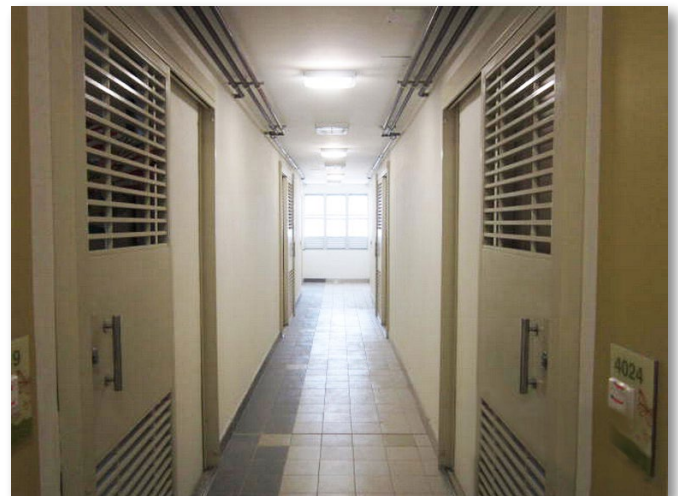
LED installations at Kai Ching Estate
