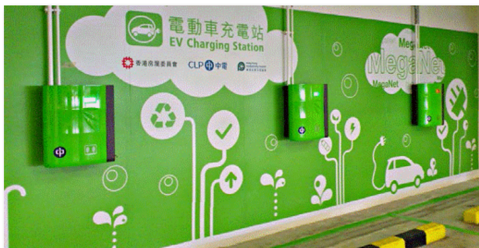
EV charging facility at Choi Tak Shopping Centre Carpark
