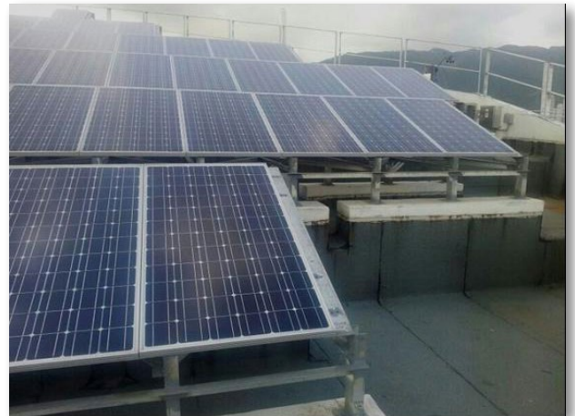
Solar panels at Kai Tak Site 1A
