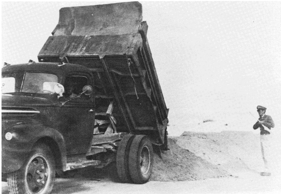
Figure 12. Pouring gypsum for road shoulder construction (1930s). (Courtesy White Sands National Monument)
