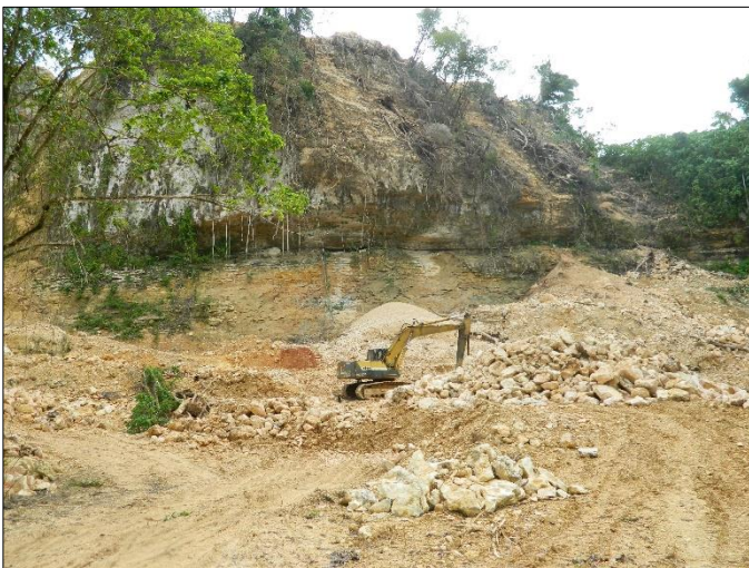
Fig. 3. A new limestone quarry to supply local road construction materials, Oikull, Airai State, Republic of Palau.
