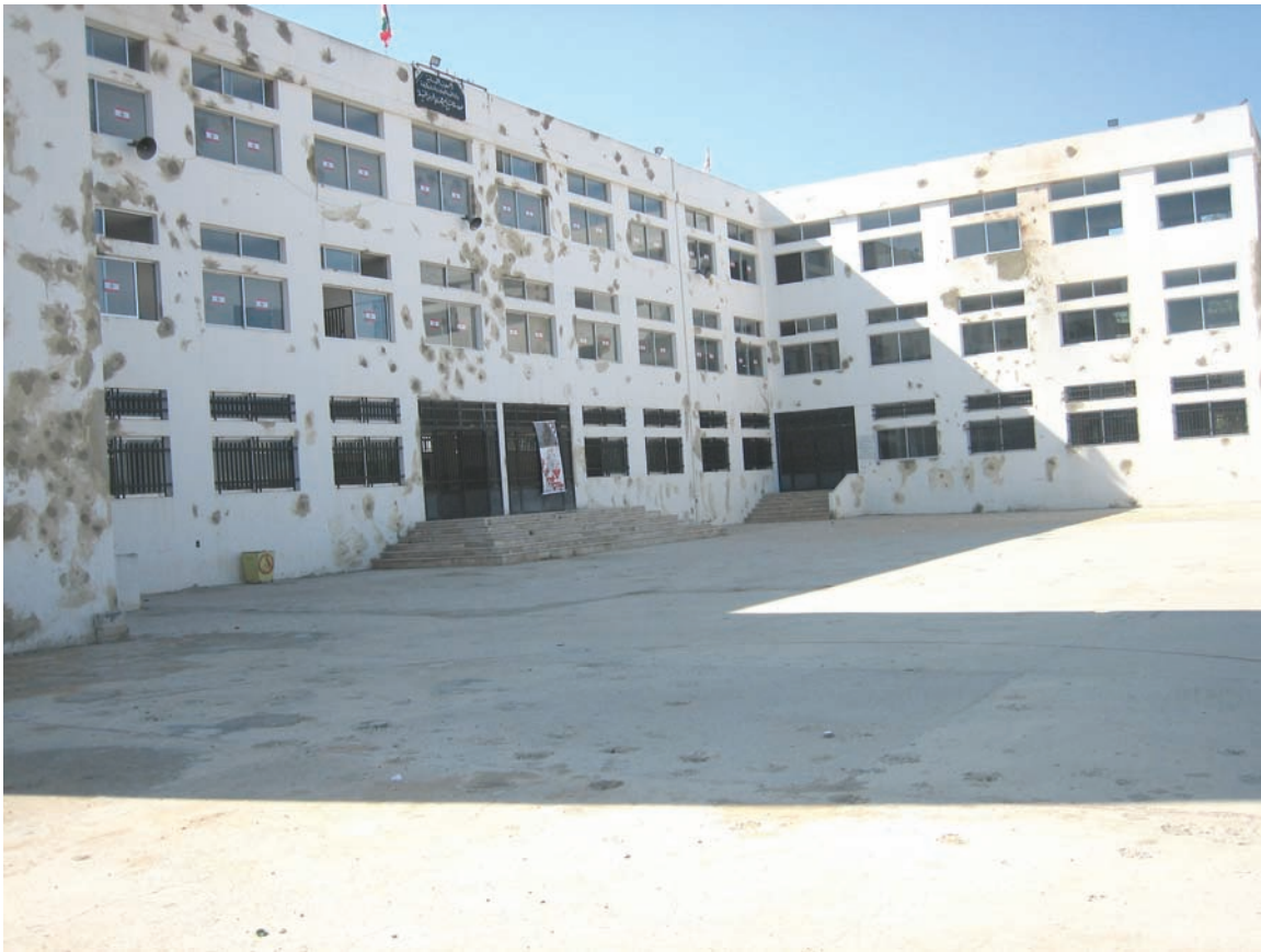
Al-Sheikh Naïm Mahdi primary school in Zawtar al-Sharkiyeh exhibits the typical pockmarked walls of a building struck by cluster munitions. On October 23, 2006, the municipal leader said that deminers had removed 2,000 to 3,000 submunitions from the property. © 2006 Bonnie Docherty/Human Rights Watch
