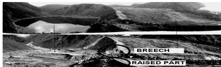
Figure 2 the photo shows the raised part of the dam, the breach at the abutment and the silt accumulated in the dam (WIHG).
