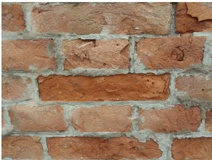
Figure 20. Brick masonry of an old factory converted to a modern building. The OPC cement used to repoint the joints is deleterious in terms of rigidity and salt leaching.
