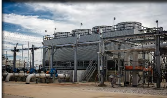
Figure 13-5. Mechanical draft cooling tower
