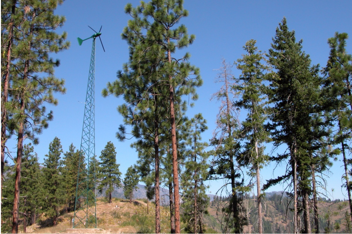
Figure B-2. Grim turbine in Peshastin, Washington. Photo by Abigail Krich, NREL 13495
