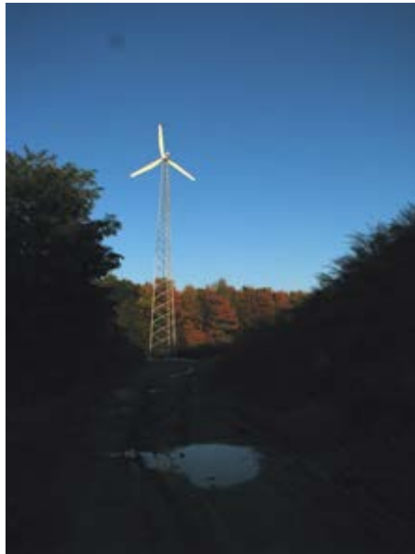
Figure B-4. Turbine in Kittery, Maine. Photo by Donald Doval, NREL 28427
