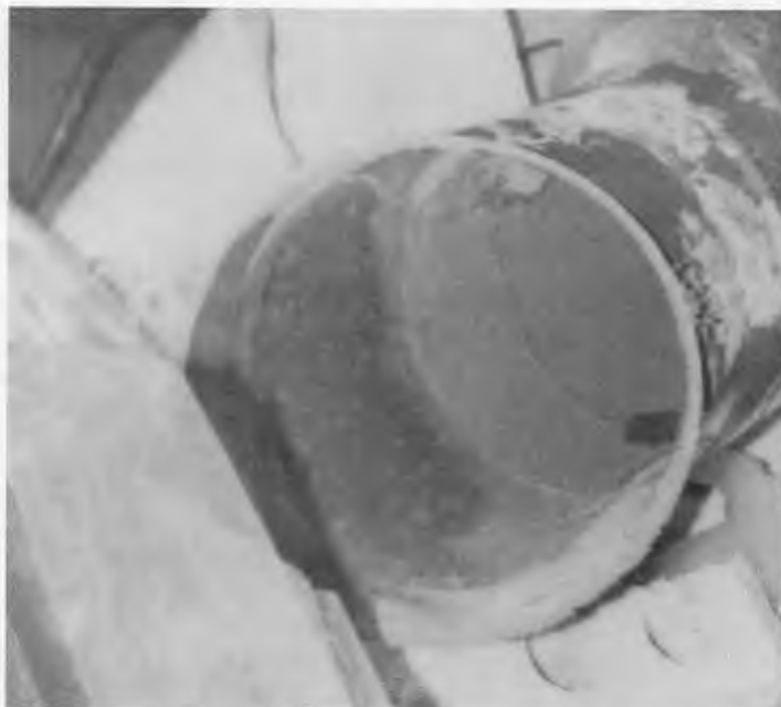
Perchlorate salt deposits are visible on the inner walls of this duct elbow of a laboratory hood.
