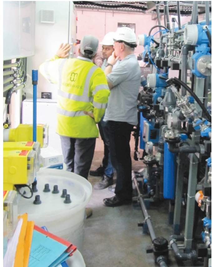
Figure 4: Prototype plant in Ahmedabad
