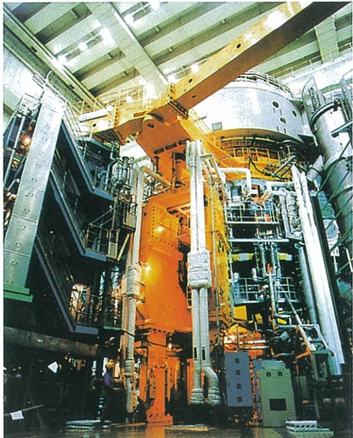
JT-60: Large tokamak device
