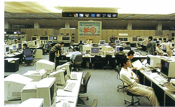
JT-60 central control room
