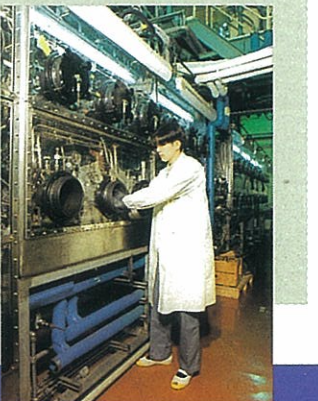
A tritium handling system with glove box
