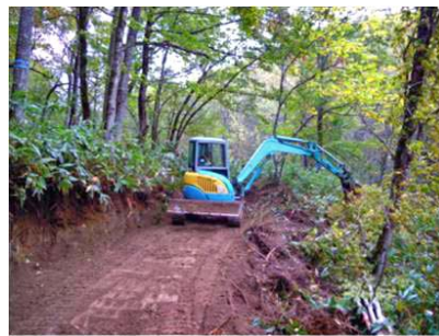
Construction of a “forestry operation road” for forestry machinery such as forwarders (National forest in Shibetsu-shi) [Kamikawa Hokubu District Forest Office]
